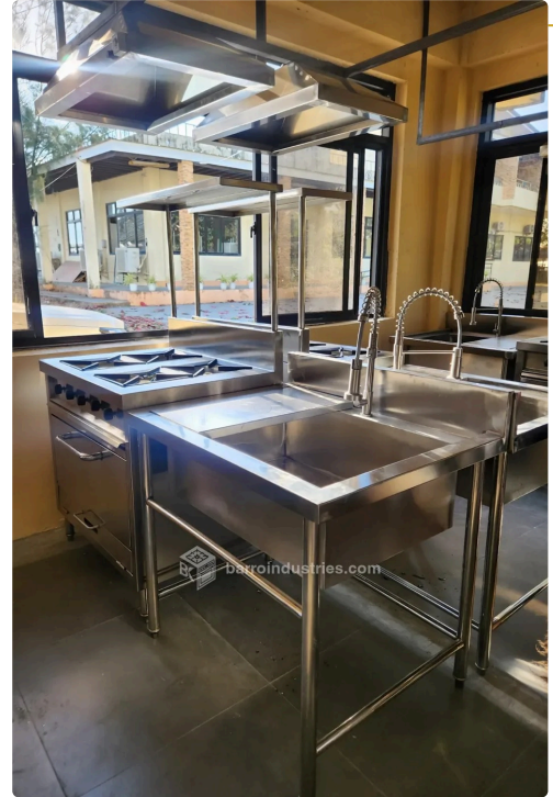
A sink station with an overhead shelf, installed at ISPSC.
