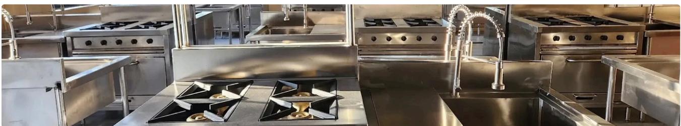
A gas range and sink at ISPSC (March 2026).
