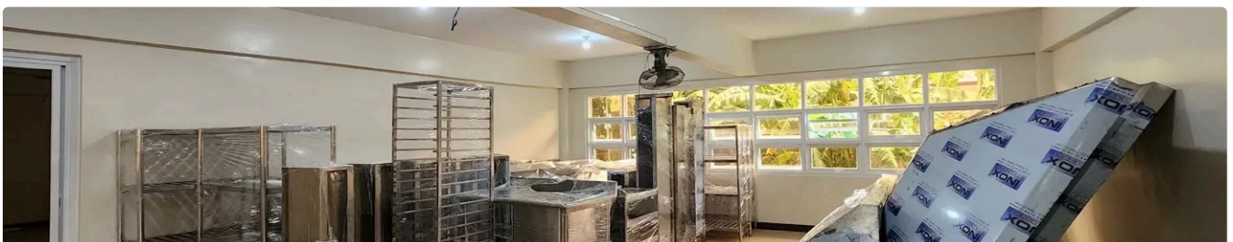
DMMSU: installed stainless-steel tables and racks, wide view
