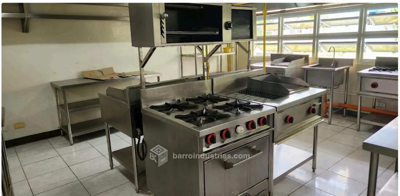
DMMMSU: finished commercial kitchen with range, hood and work tables
