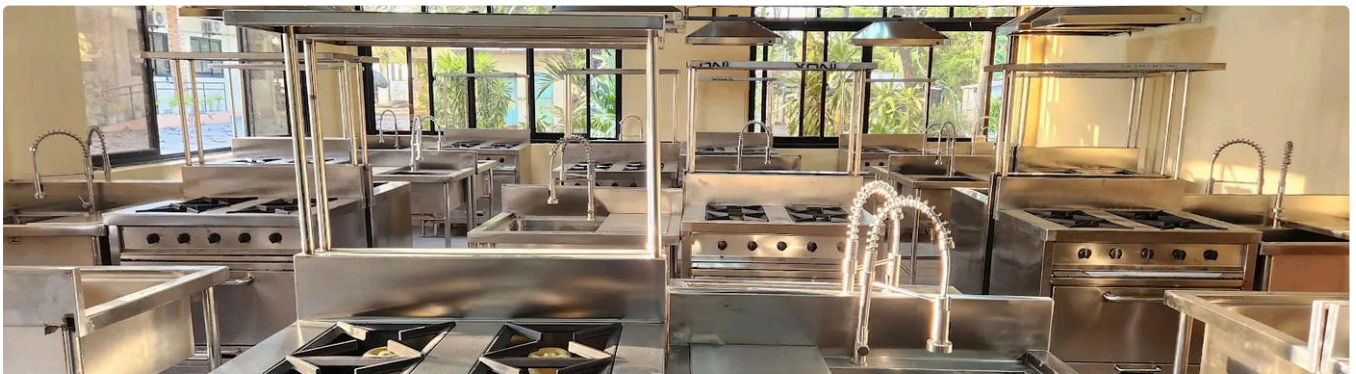
ISPSC 2026: wide view of the cooking stations with range ovens, sinks and overhead hoods
