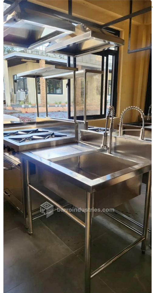
A sink station with an overhead shelf, installed at ISPSC.
