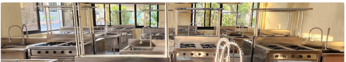
Cooking stations with range ovens, sinks and overhead hoods at ISPSC.
