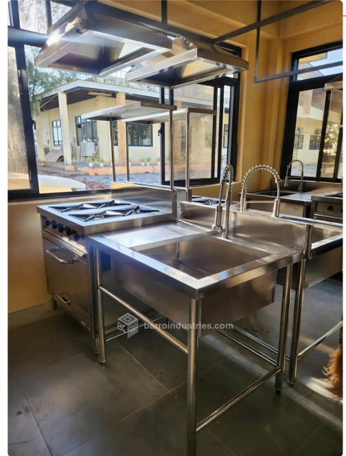
A sink station with an overhead shelf, installed at ISPSC.
