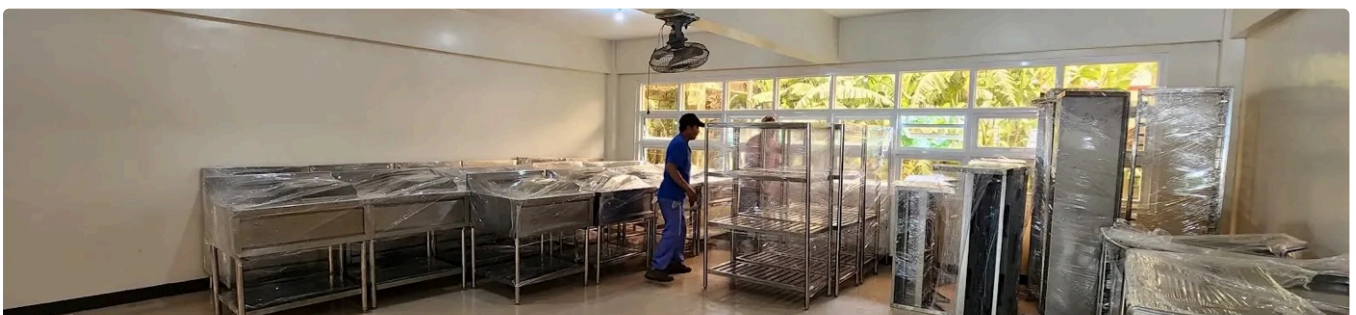
DMMMSU: room installed with stainless-steel tables, racks and shelving
