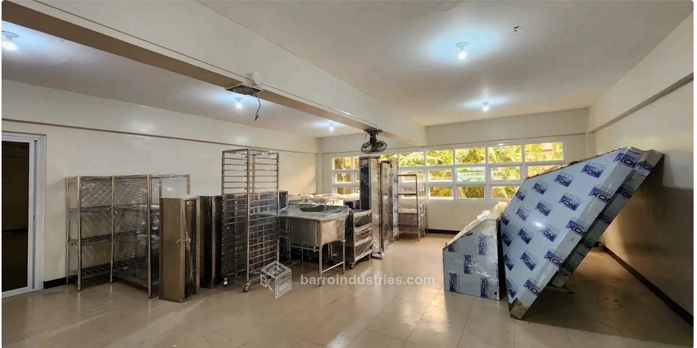
DMMMSU: installed stainless-steel tables and racks, wide view
