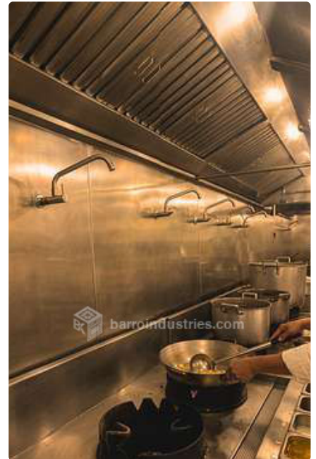
Cooking at the line, under the hood.
