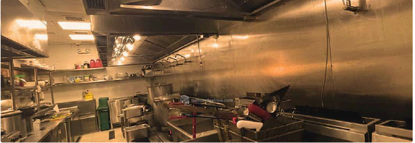
The cooking line along the stainless-steel wall, under the exhaust hood.
