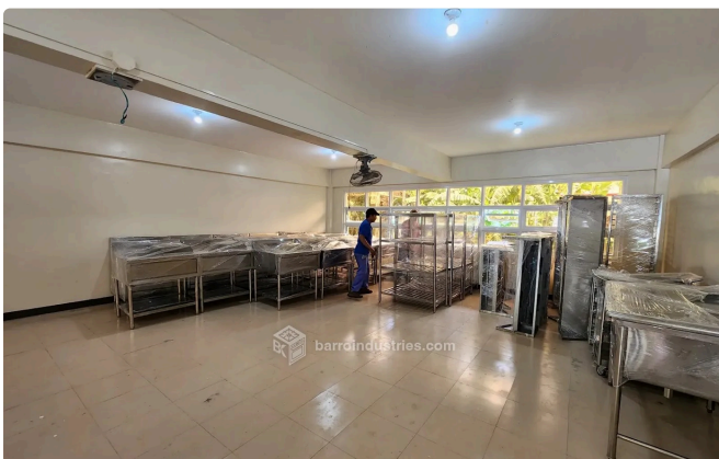
DMMMSU: room installed with stainless-steel tables, racks and shelving
