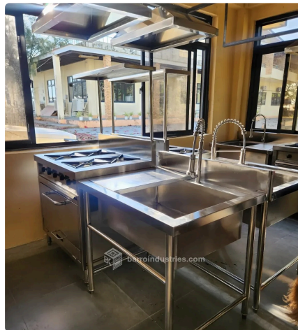
ISPSC 2026: sink station with an overhead shelf
